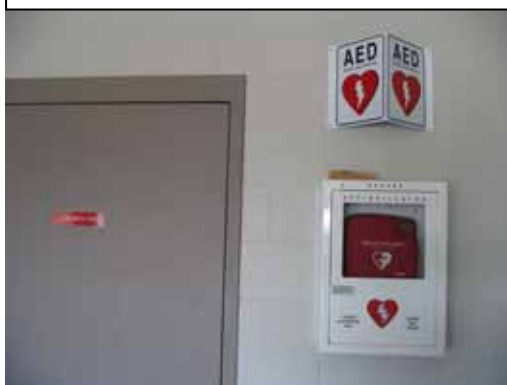
Ag Complex main hall by Communications Room
